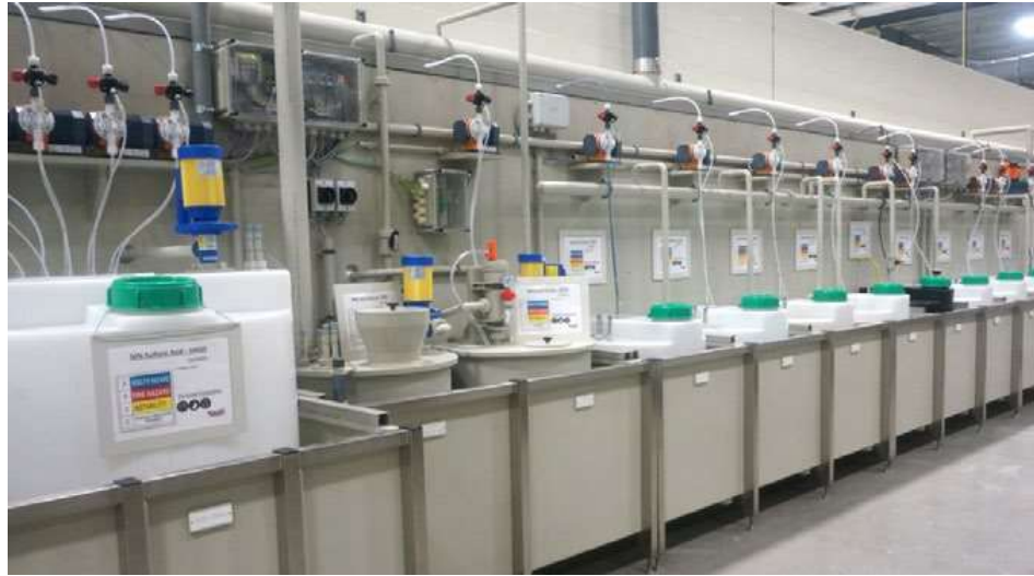
Chemical dosing stations.
