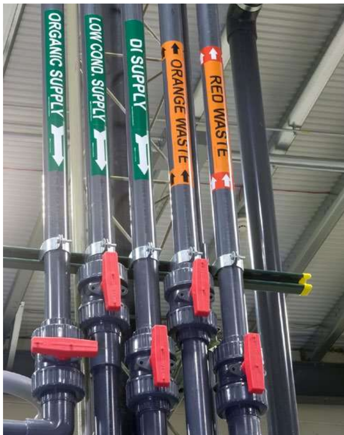
Detail of custom piping.
