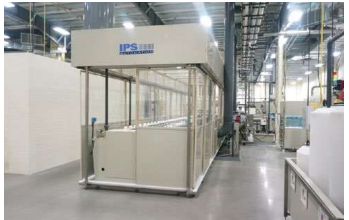
Fully automated IPS ENIG plating line.
